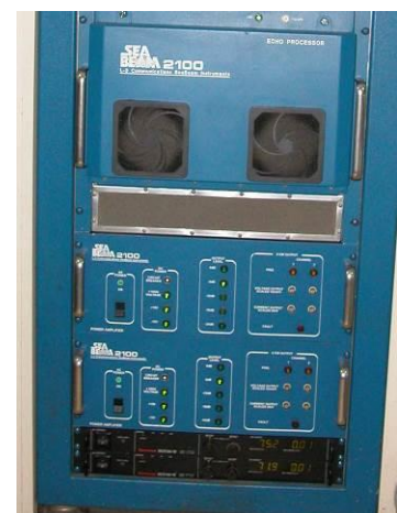
Figure 12: SeaBeam 2120 system electronics cabinet.
